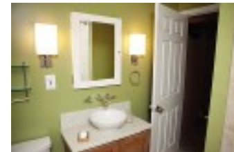
AFTER: After gutting the entire space, the room got a fresh coat of paint, a deep tub, an energy-efficient toilet, a ceramic-tile floor and a new vanity/sink. Now the bath has an open feel and a beautiful, finished look.
